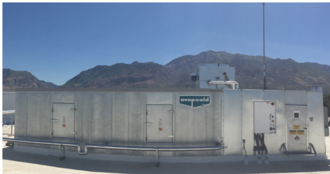
One of two Evapcold LCR units, fully installed at Western Gateway.
