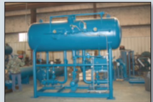
Liquid recirculator package with pumps and controls
