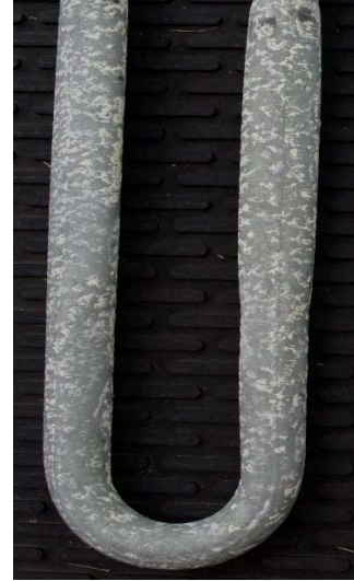
White rusted coil
